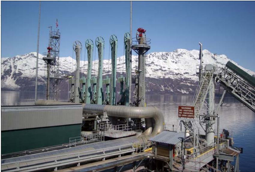
Image of berth 5 showing oil and ballast water pipes—image taken by Mark Morones
