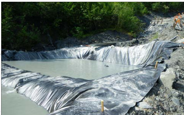
Containment material put in place to protect surrounding area. Photo taken by Justin Selvik, Natural Resource Specialist III, JPO/SPCO.
