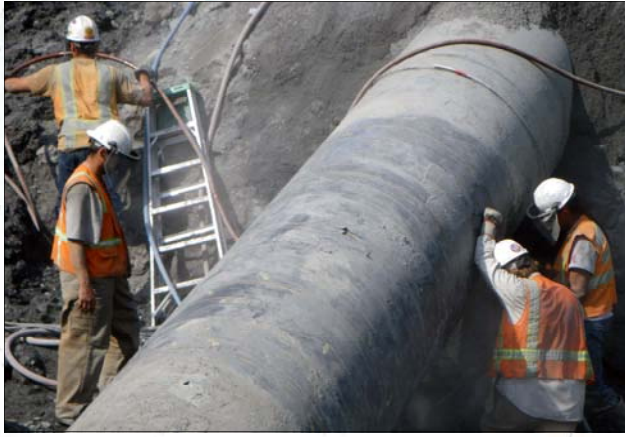
Alyeska employees working at pipeline mile post 792.5 to remove a large rock structure that had been pressing against an underground segment of the Trans-Alaska Pipeline. Photo taken by Justin Selvik, Natural Resource Specialist III, JPO/SPCO.
